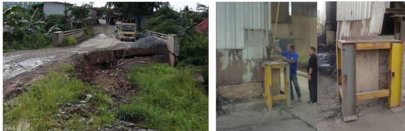
(a) The bridge embankment landslides (b) Shifting column
