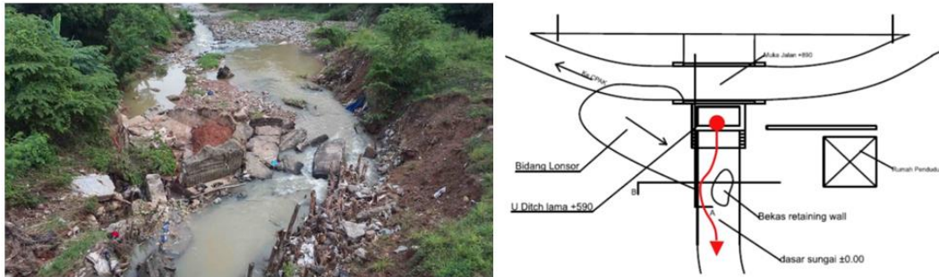
(a) The remnants of the bridge wing wall in the river. (b) The downstream turns sideways and erodes the bottom of the bridge embankment slope
