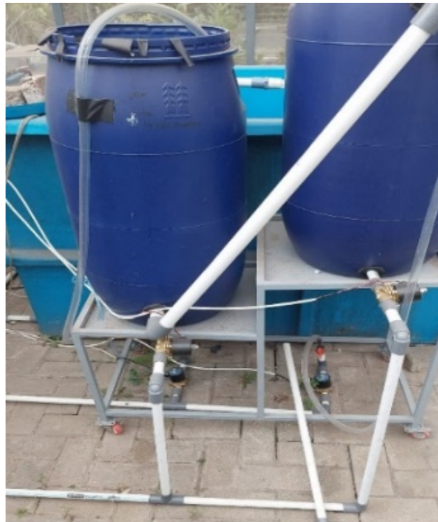
Fig. 4. Design of the filtration system and measurement experiments conducted at Telkom University
