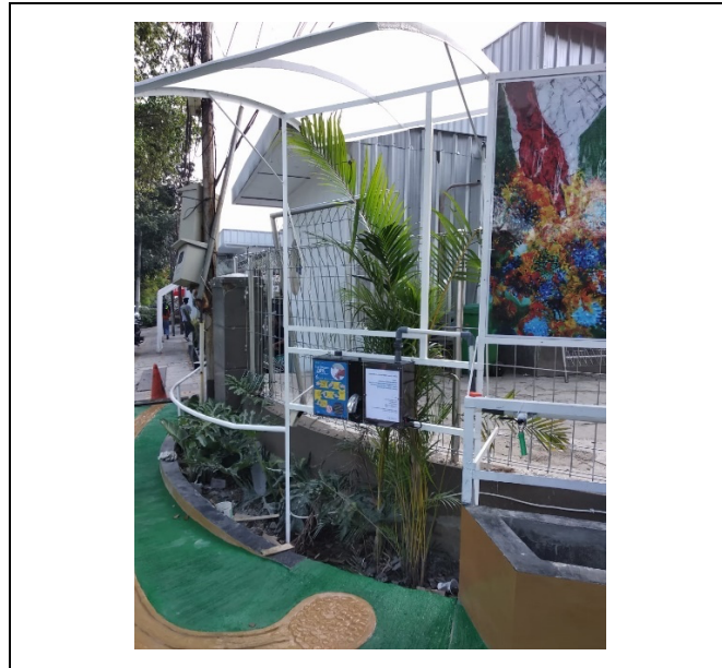
Fig. 6. A touchless automatic hand washing machine installed on Jalan Geusan Ulun , Bandung
